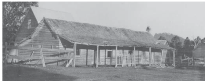
The original Bankfoot House, 1926. At this time the log foundations were rotting and the building deteriorating. The slot of the post box is visible in the centre of the front wall. This photograph illustrates the relationship between the two buildings. The new building's steep pitched roof is showing at the rear of the old building.
